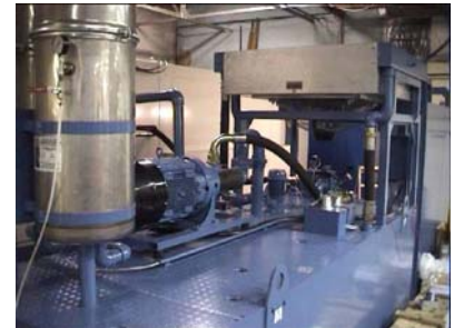
Special filtration to suit application. Unit shown is a cartridge system fitted with a 300 litre / min triple screw pump to feed the application oil and a fan cooler to maintain oil temperature
